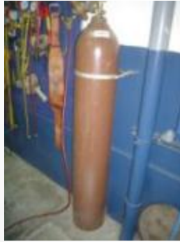
DRY NITROGEN EQUIPMENT
